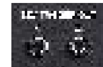
12v out jacks
